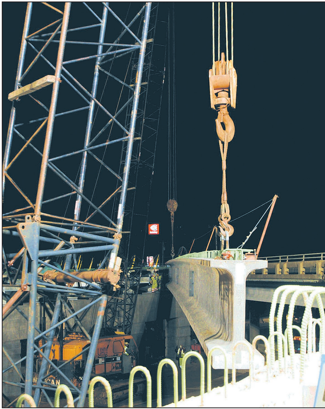
PHOTO BY GREG GRANGER The weather finally cooperated, and E&J Construction, working for general contractor Lunda Construction Co., lifted the remaining prestressed concrete beams into place on Anoka County's new Lake Drive bridge over I-35W in Lino Lakes last Thursday night. Federal and state approvals have just launched the second new interchange in the city, planned for construction in 2009 on the Lino Lakes/Hugo border (see story this page).
